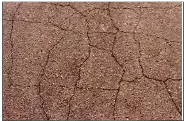
Condition 5 – Very Poor
